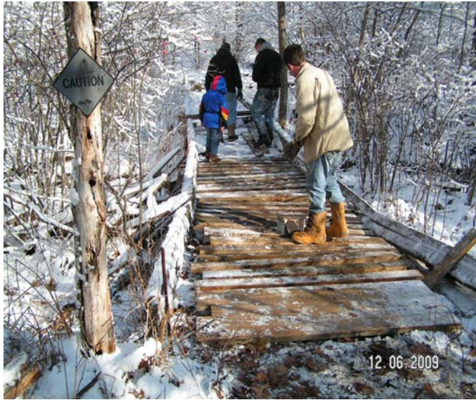
Shown above are from left Owen Shattuck, Larry Tucker, Job Shattuck, Ed Morrin with photographer: Andy Katafiasz who worked to repair the “Bridge at Partridge Hollow” on the Trail North.
